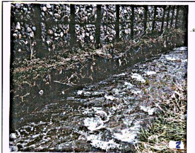
Figure 6. Sidewall damage by high velocity flow
