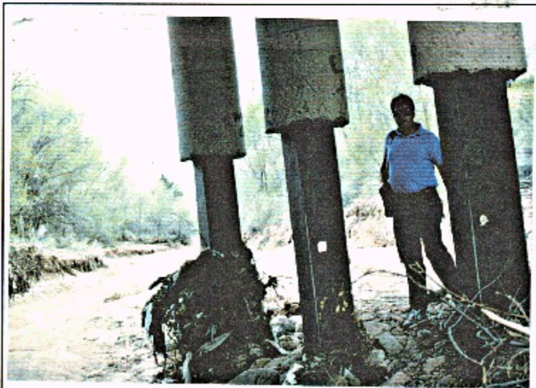
Figure 22. Public confidence can erode with the channel bed.
