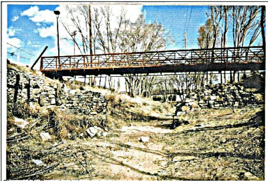
Figure 14. Breached check dam
