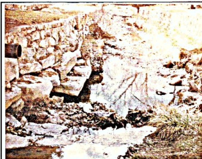
Figure 15. Undercutting below grade control
