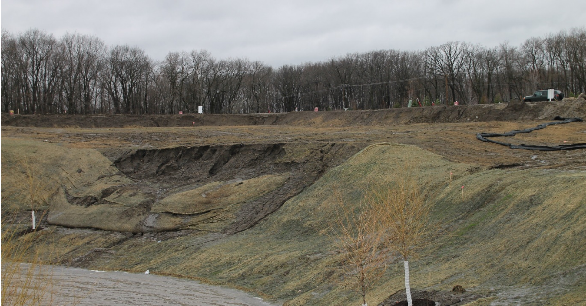
Figure 21: Typical slope failure
