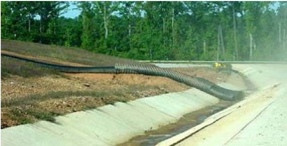
Figure 15: This storm drainage pipe empties into a drainage ditch. Controls both run-on and run-off
