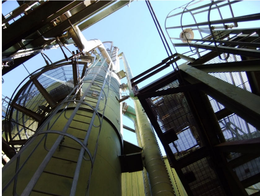
Figure 17 View looking up at amine contactor tower at a major oil and gas company natural gas treating facility.
