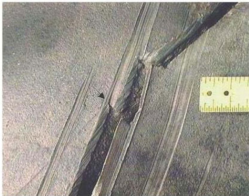
Figure 2 Fracture origin (arrow) and gouges that caused brittle fracture failure on 20-inch OD carbon steel pipeline [8].
