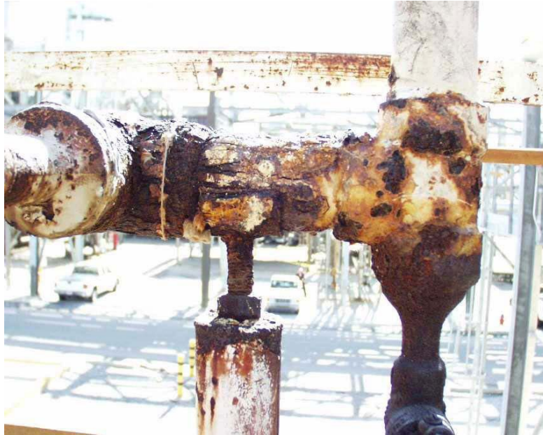
Figure 7 Insulated liquid level bridal with CUI [8].
