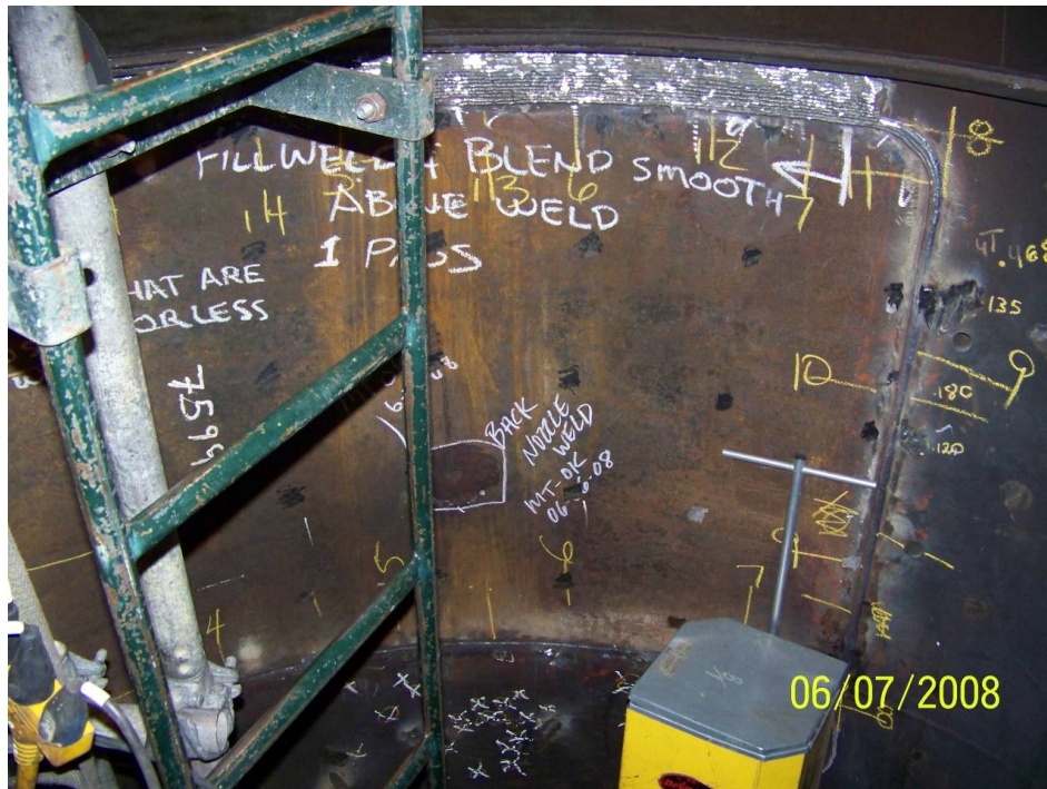
Figure 42 Photograph of flush patch and weld build-up from inside of amine contactor tower. Photograph courtesy of Sandstone Engineering in Farmington, N.M.
