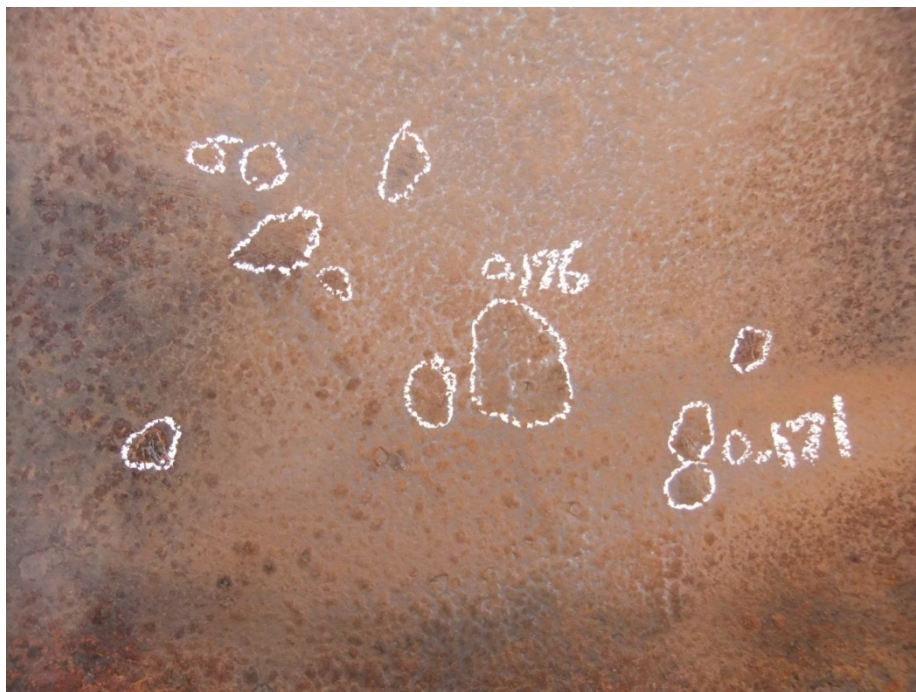
Figure 21 Pitting identified during internal inspection of pressure vessel.
