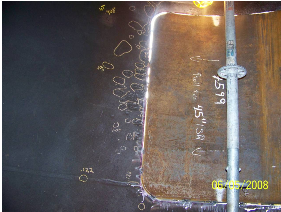
Figure 41 Photograph of fit-up of flush patch from inside of amine contactor tower and adjacent pitting. Photograph courtesy of Sandstone Engineering in Farmington, N.M.
