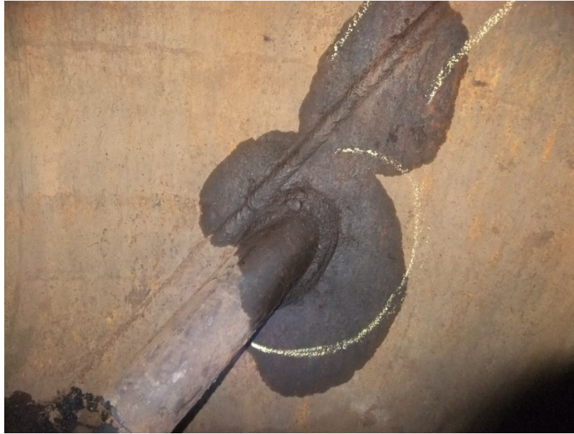
Figure 39 Internal visual inspection showing post WFMT inspection of nozzle internal weld. Courtesy of Sandstone Engineering in Farmington, N.M.
