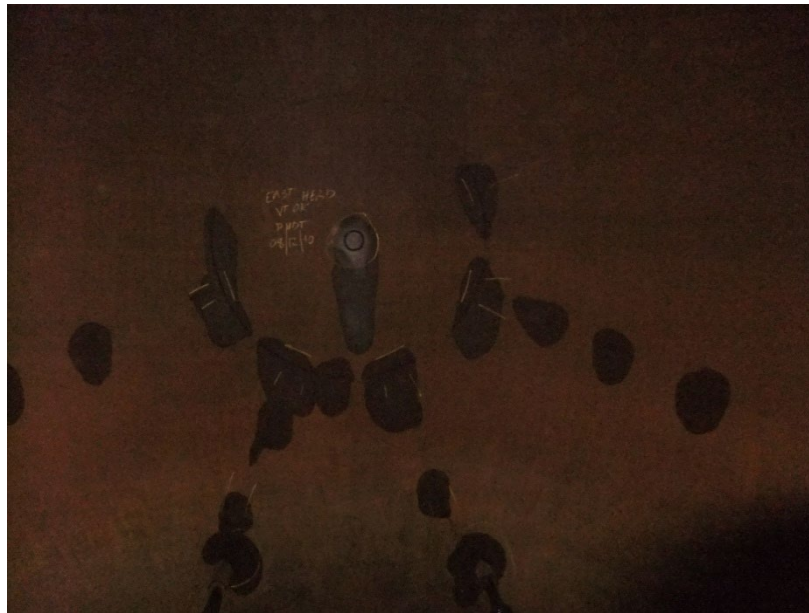
Figure 38 Internal visual inspection showing post WFMT inspection of ~30% of hemispherical head welds.
