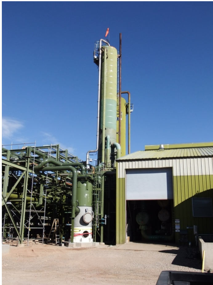
Figure 16 Amine contactor tower at major oil and gas company owned natural gas treating facility.
