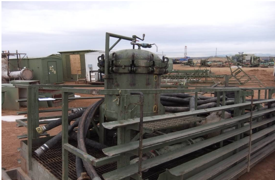
Figure 19 Filter Specialists, Inc. sock filter vessel on portable skid used for filtering water in natural gas drilling operations for a major oil and gas company.
