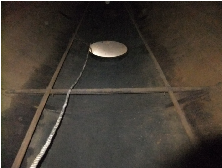
Figure 24 Internal view after internal inspection on bottom of bullet tank at a major oil and gas producer's natural gas processing facility.
