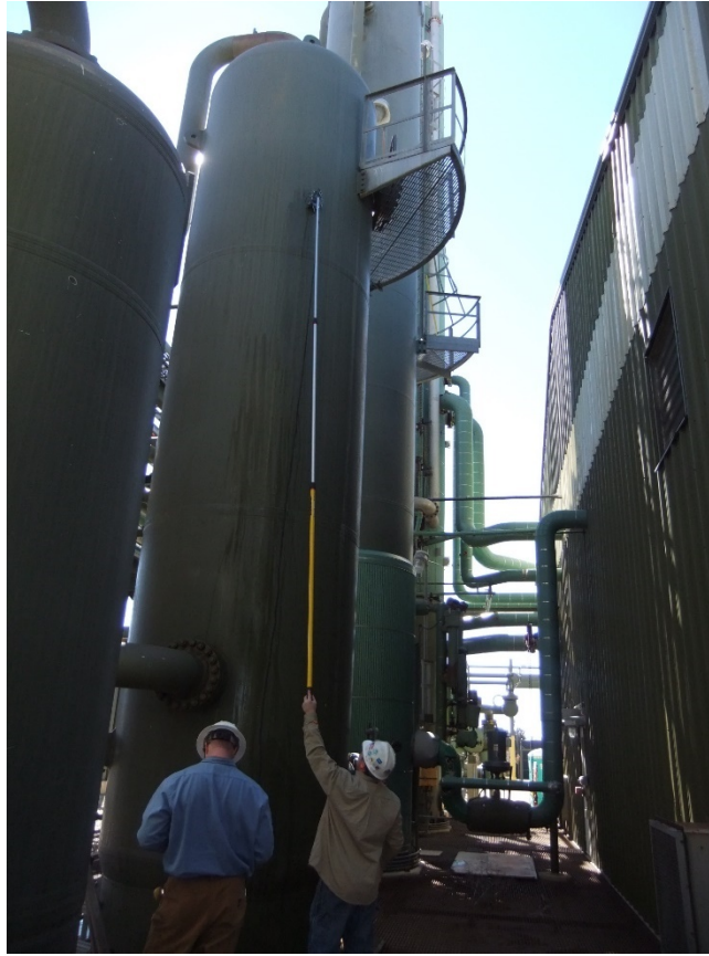
Figure 31 View of manual UT crawler on pressure vessel tower, courtesy of Sandstone Engineering
