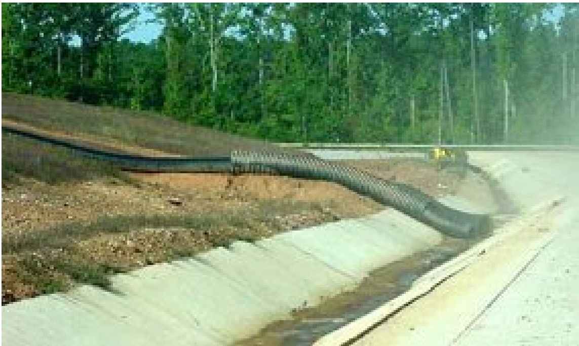
Figure 40: This storm drainage pipe empties into a drainage ditch. Controls both run-on and run-off
