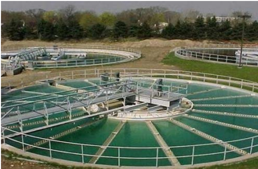
Circular settling tank with radial weirs 2
